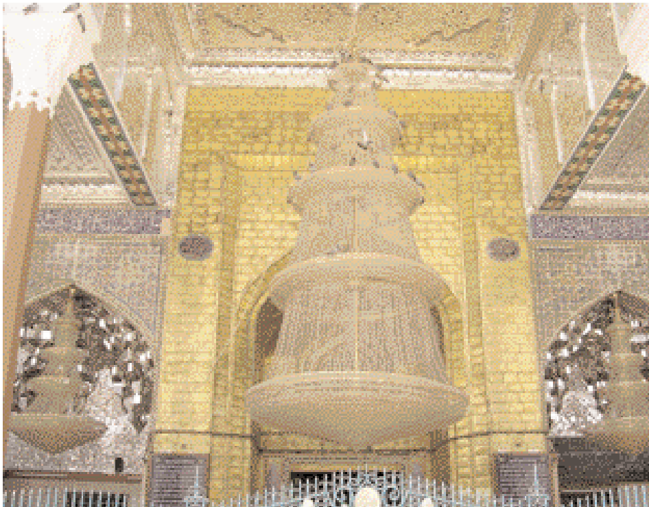
Precious chandelier covered because of the on going repairs in the shrine
